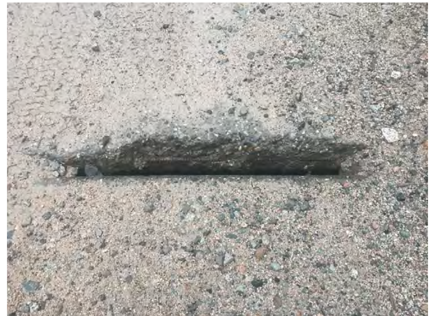
Damage at left approach
