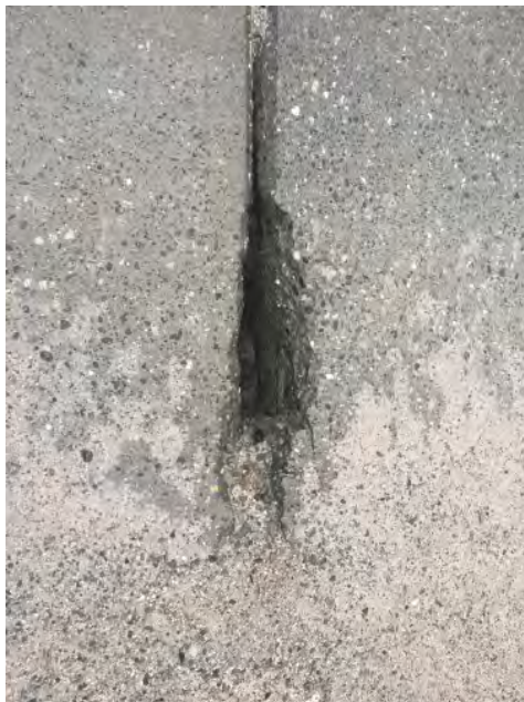
Damage to deck panels
