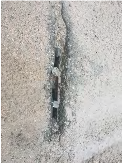
Damage to deck panels
