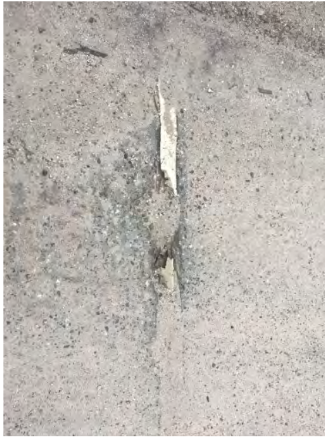
All deck joint seals gone
